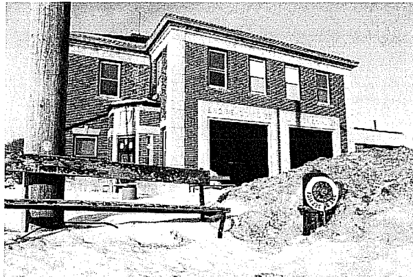
Broken hydrant outside of a Detroit fire station for Engine 55 and Ladder 22. Steve Neavling/MCM
